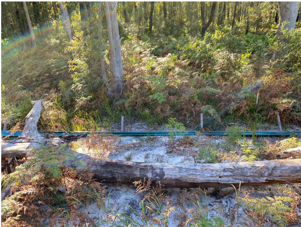
Photo 14 – Sediment fencing is down in a couple of small areas
