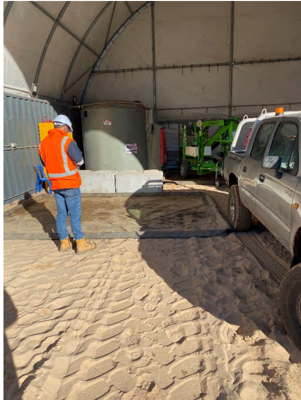
Photo 1 – Portable Bund for Maintenance Activities
